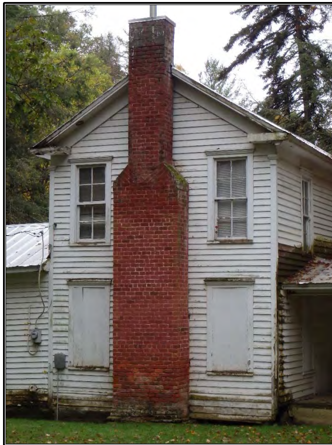
Figure 42. Detail view of the brick end chimney of the Frank Seagraves House (AH0191), facing southeast.
