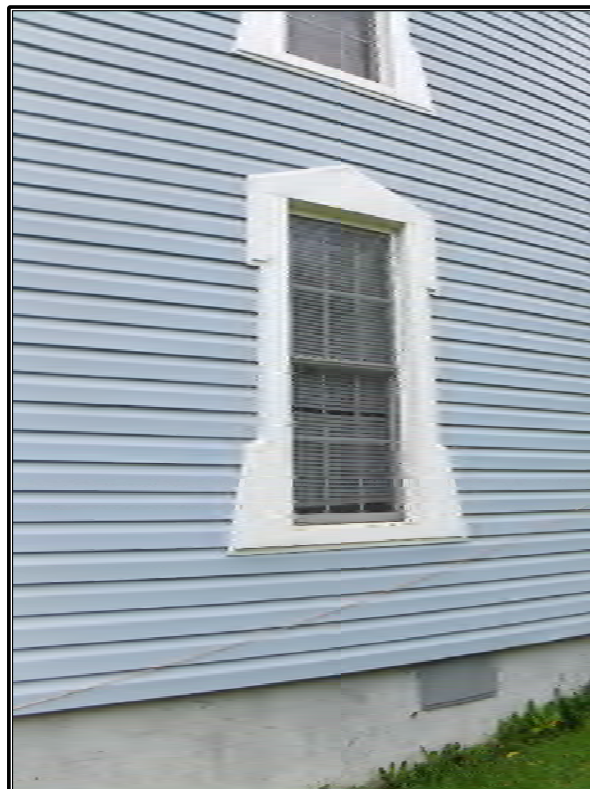
Figure 52. Detail of an aluminum-clad window surround on the north elevation of the Frank Edwards House, facing southeast.
